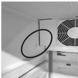
From the inside the cabinet
